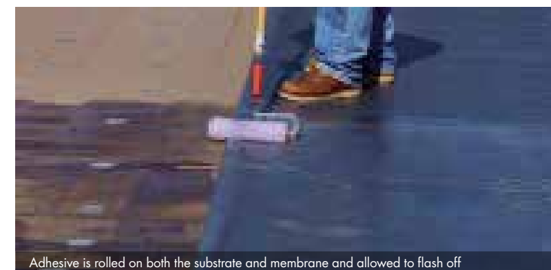
Adhesive is rolled on both the substrate and membrane and allowed to flash off
